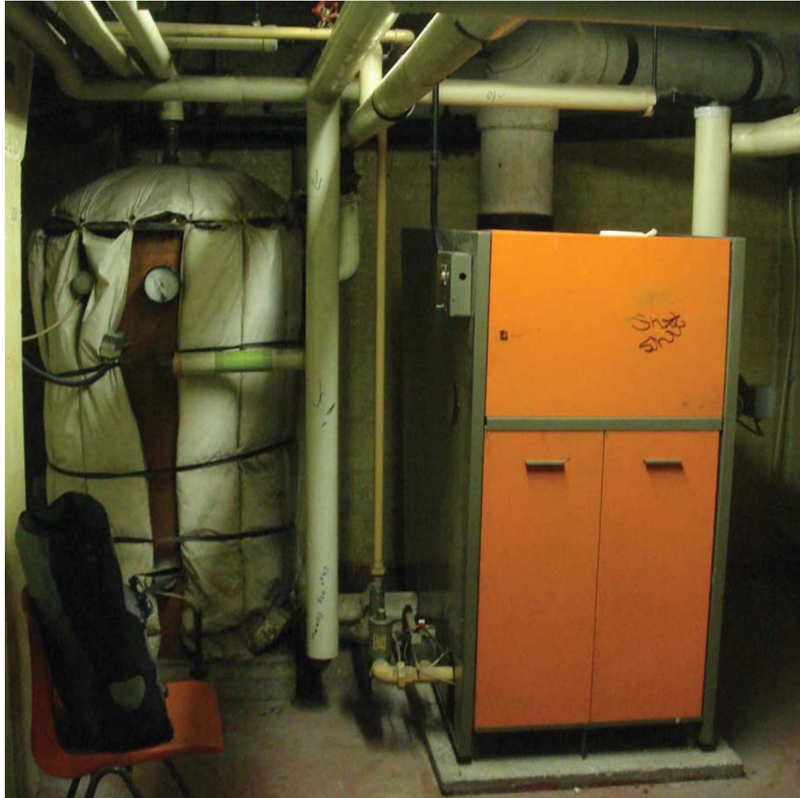
Gigantic gas boiler and virtually un-insulated tank
