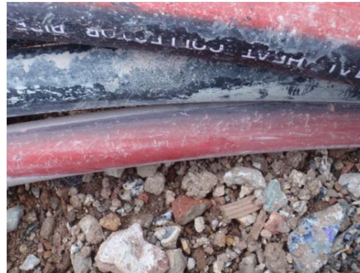
Upper pipe after test
