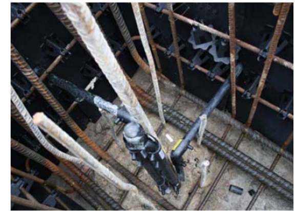
Cage and header pipes
